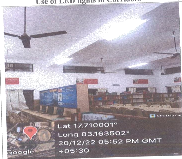
Use of LED lights in Library
